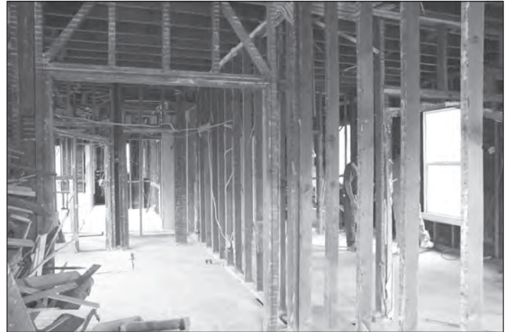
Laura's Place - down to the studs in preparation for electrical work and new drywall.
